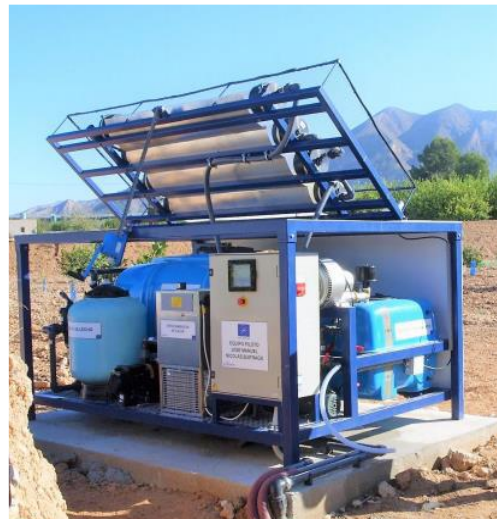
Pilot photocatalytic plant installed at Finca Torreblanca, Torre Pacheco, Murcia, Spain ( http://www.life-aquemfree.eu/ )
