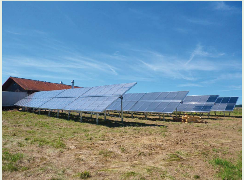
Solar thermal heating of gas pressure control systems in Großseelheim, Germany
