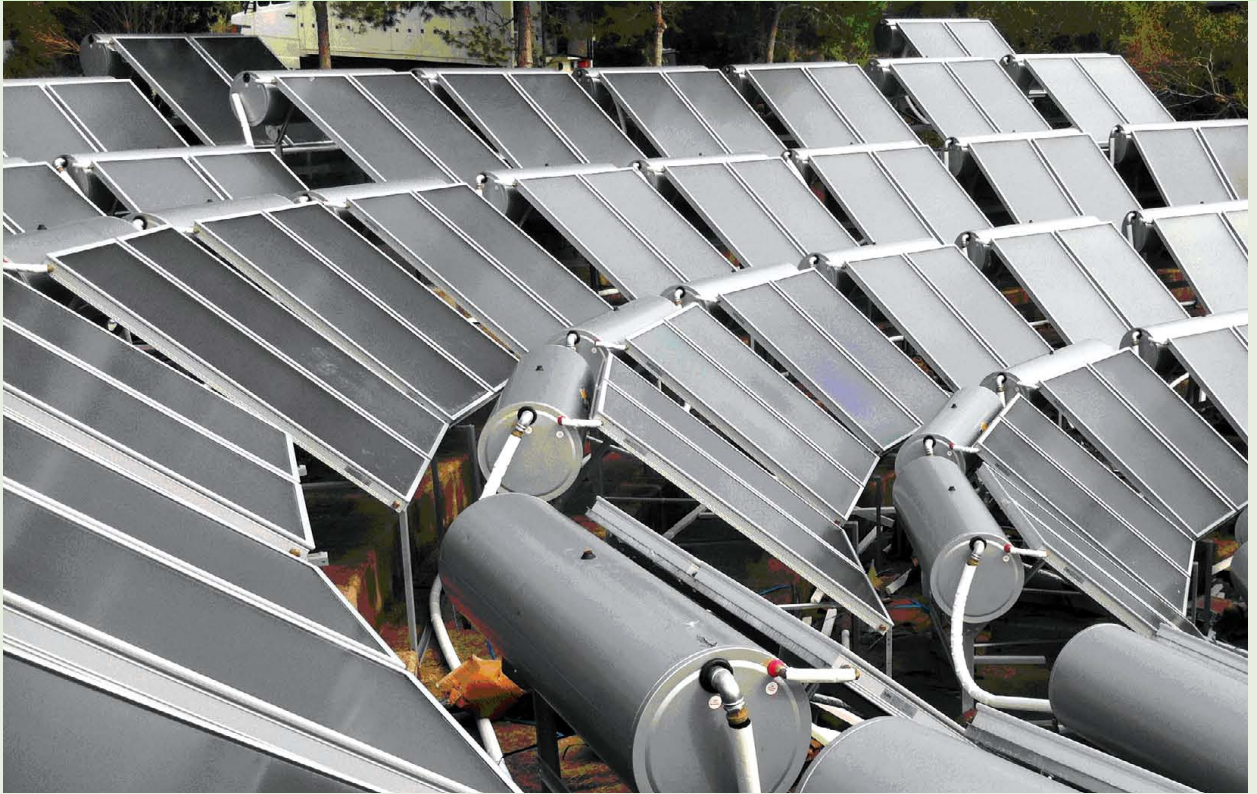
Greek thermosiphon systems
