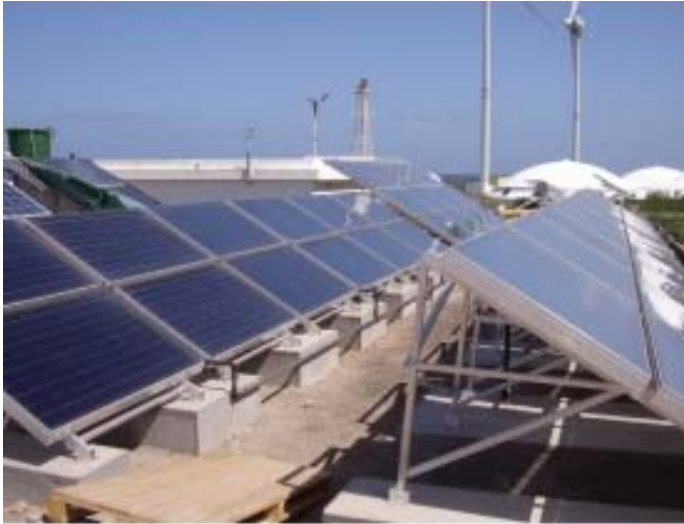
Sea water desalination Gran Canaria, Spain (Fraunhofer ISE, Germany)
