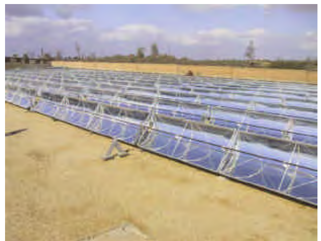
840 kW solar thermal plant for a chemical industry in Egypt
