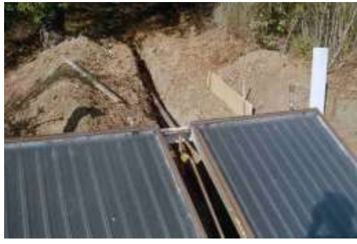
Figure 34. Classic Thermosyphon Pipes above The Collectors.
