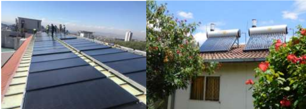
Figure 3: PVT demonstration system installed by Greenline Africa at a hospital in Cape Town, South Africa (left) and two thermosiphon systems with ETC at CPS sisters' youth hostel in Harare, Zimbabwe. Photos: Solarus Smart Energy Solutions (left), Werner Weiss, AEE INTEC (right)
