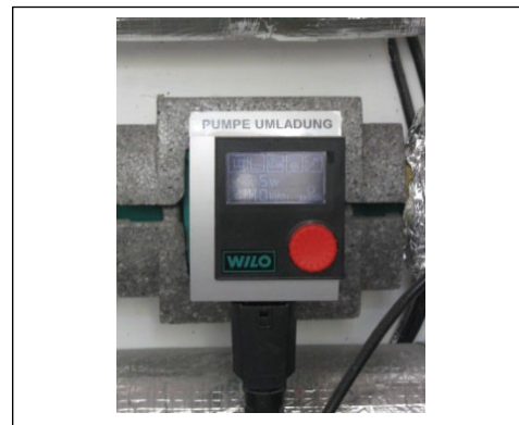
Figure 25: Transfer pump in operation
